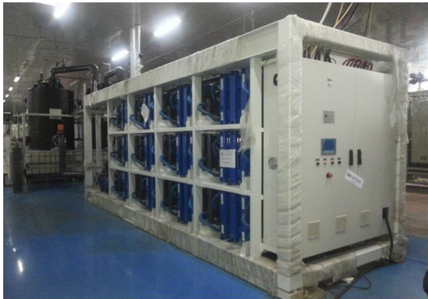
Each Power Module is composed of 12 stacks, pumps and controls. Tanks and power conversion system (PCS) are separate based on system energy rating.
